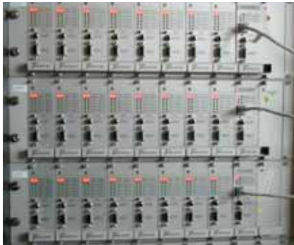
8 VIP boards integrated into a standard 19" rack.
