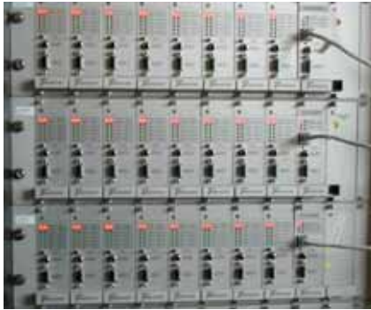
8 VIP boards integrated into a standard 19" rack.
